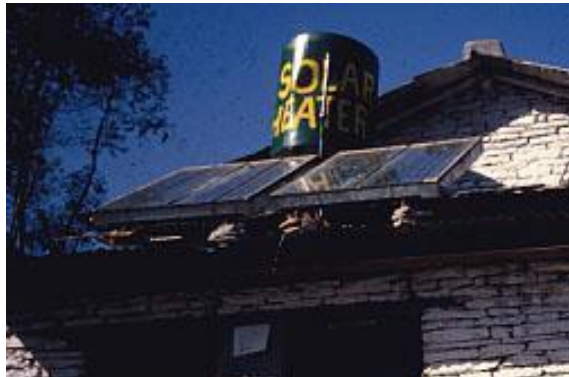
Figure 6: Solar water heaters in Nepal. Photo: Practical Action.
